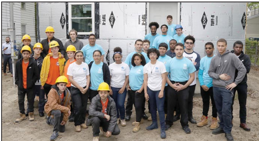
A partnership of the Roger L. Putnam Technical Fund and the Greater Springfield Habitat for Humanity enabled the carpentry students at the school to help build a house at 101 Orchard Street. The project is a culmination of their first-year partnership.
